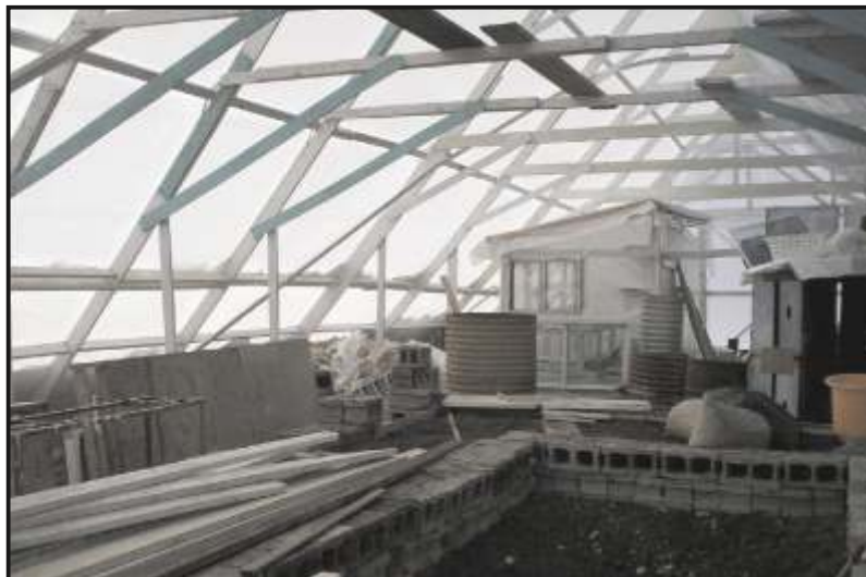
Interior of A-frame, still under construction, showing small interior starter greenhouse, which warmed up to 68 degrees F inside, by solar heat alone, despite the wind-chill factor outside, and the ice on the inside walls of the big A-frame. This will allow us to start seedlings earlier in the spring and heat only at night. We may find that we can simply cover the seedlings at night in spring and not have artificial heat out there at all. See article.
